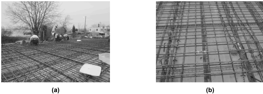
Figure 10 – Instrumentation for Concrete Bridge Deck (a) gauge layout and (b) installed VWG
